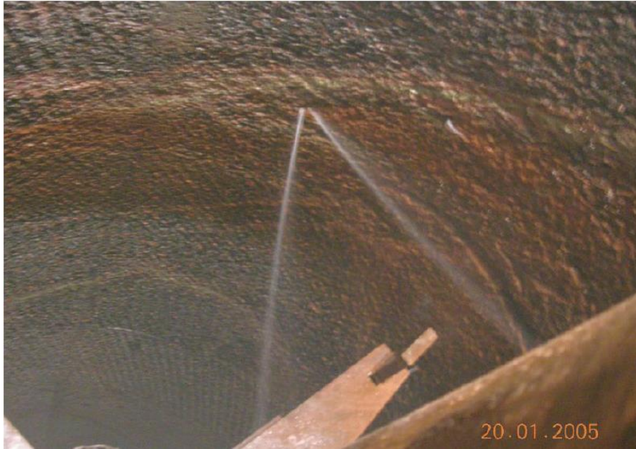
Figure 2.2. From Figure 3 in SKB-report R-05-44. Typical inflow pattern in Äspö hard rock laboratory showing high pressurized groundwater seeping out of a drilled rock surface. This photo is taken from a depth of only 220 m, i.e. the water pressure is around 22 bar, only half of that prevailing in a real repository. The cracks in the deposition holes in Forsmark are believed to be smaller but the pressure of the ground water is still 50 bar.
