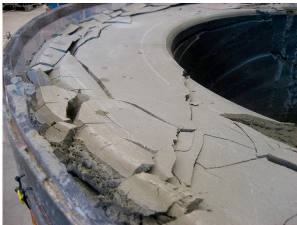
Figure 4-34. Major cracks occurred in the uppermost ring.
